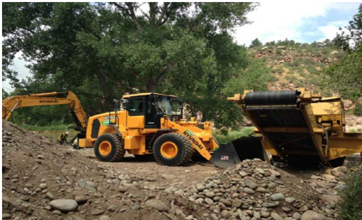
Rock screening operation for rock structures at OFC St. 2+50 and main channel St. 45+50.
