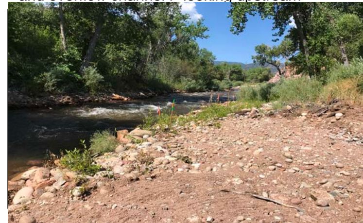
During Construction: Confluence of main channel and overflow channel F looking upstream
