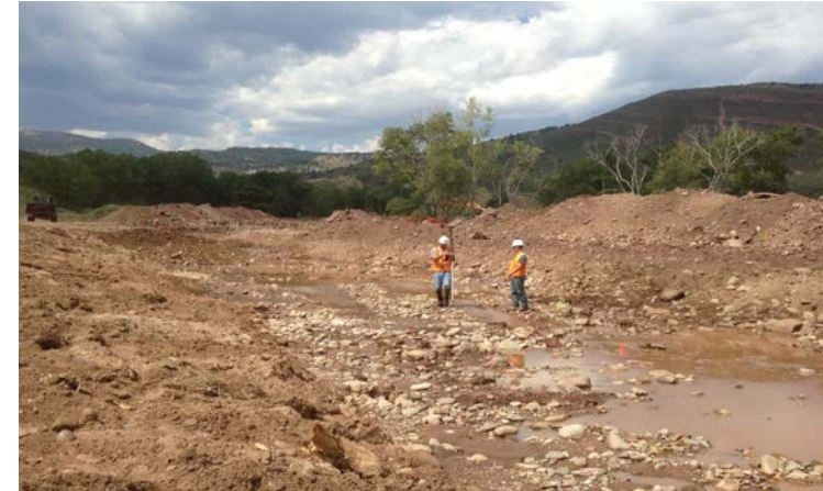
Downstream View: Mass grading of proposed main channel realignment between St. 66+50 to 77+00.
