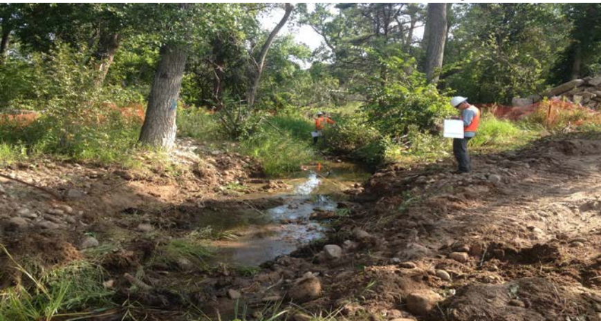
Downstream View: channel grading for Knick point stabilization rock structures in overflow channel E
