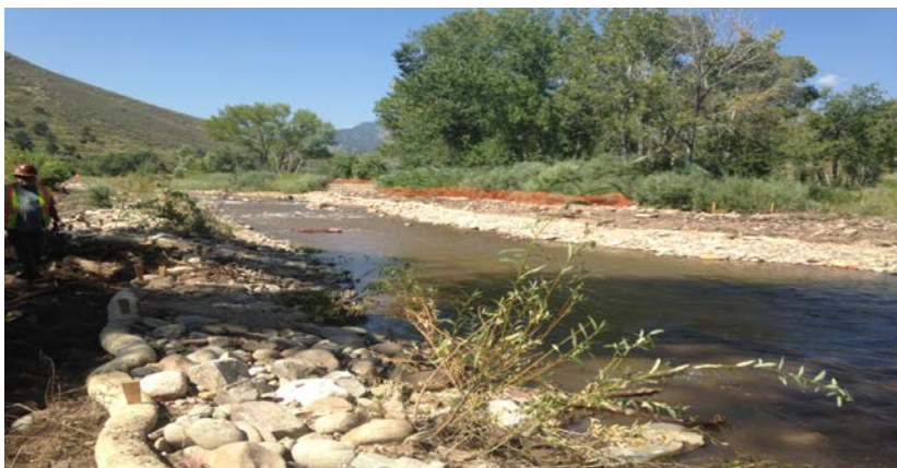
Upstream view: Fine grading and bank contours between main channel St. 60+50 to 64+00 in progress
