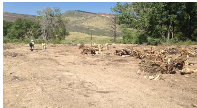
Upstream view: Installation of Type 5 Large woody structure at overflow channel C St. 7+60.
