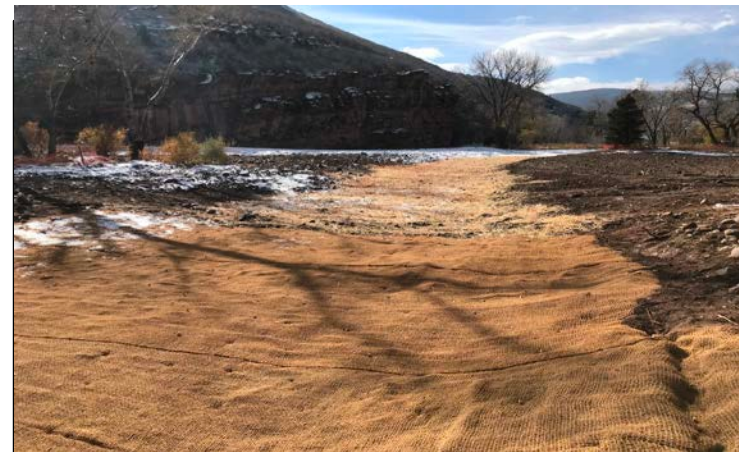
Upstream View: Erosion control blanket and wood straw mulch installed in overflow channel B.
