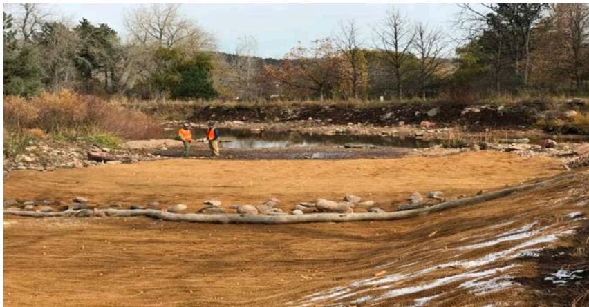
Downstream view: Installation of erosion control blankets at downstream end of overflow channel F.
