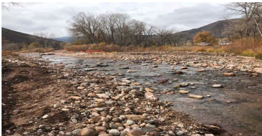
Upstream View: Completed fine grading and boulder clusters between main channel St. 74+50 to 60+50.
