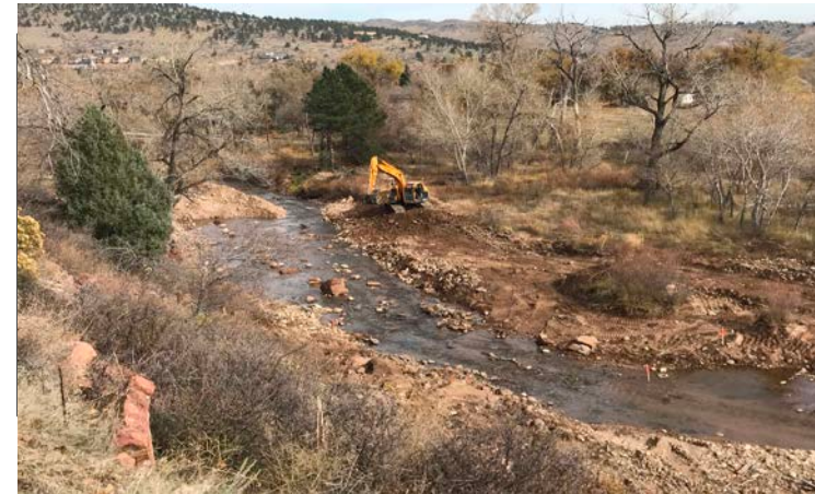
Downstream View: Right floodplain grading of SSV2 project reach between St 29+50 to 32+00
