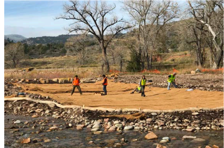
Upstream view: Installation of erosion control blankets at downstream end of overflow channel A.
