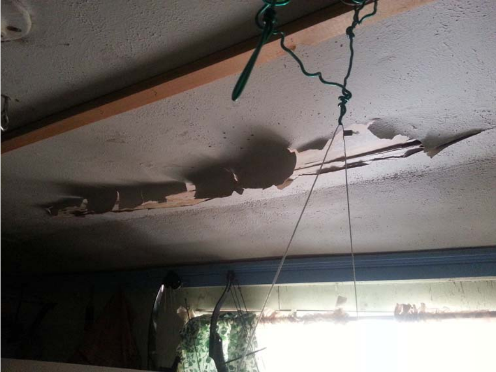
Leaking roof caused ceiling damage in kitchen
