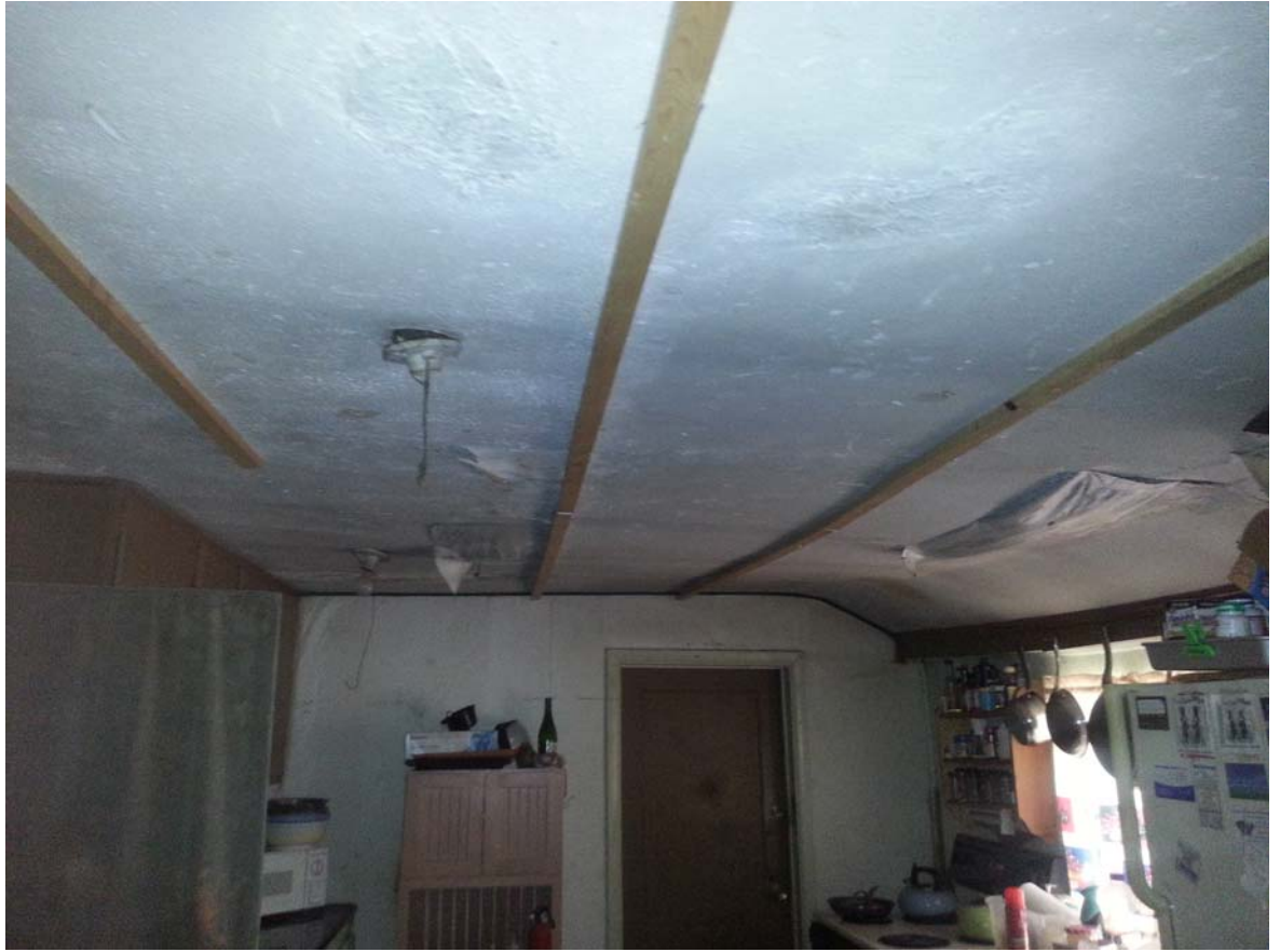
More kitchen ceiling damage
