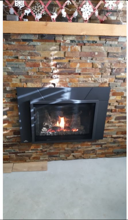
New gas fireplace.
