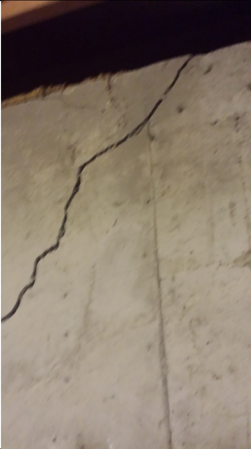
Cracks at Foundation Wall.
