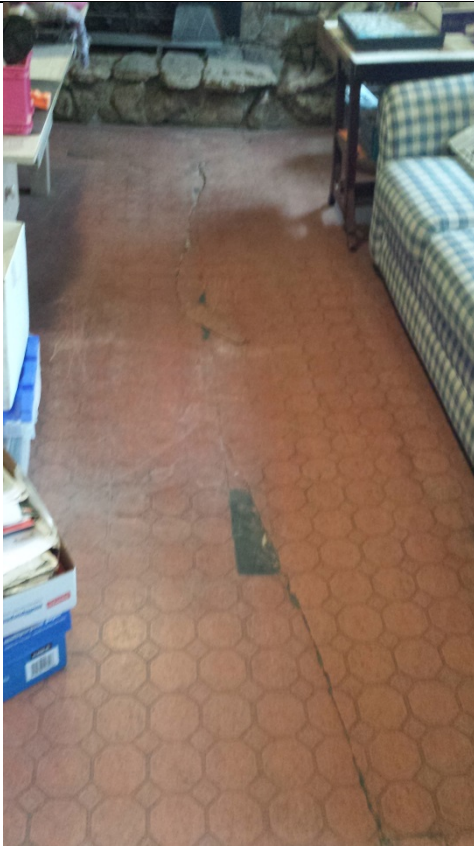
Damaged floor at family room.
