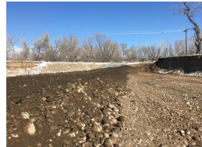
2-23-18 : Friday AM continued Breach 2 access road construction from the embankment top to the bottom of the borrow area to allow for staging of materials during breach repair
