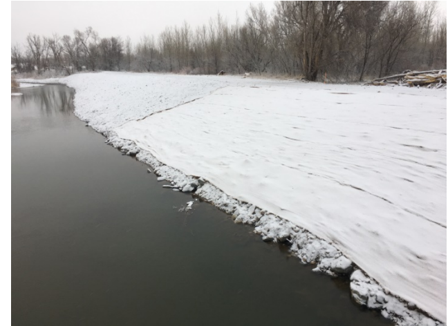
2-19-18: No further work this week on seeding and erosion control blanket installation
